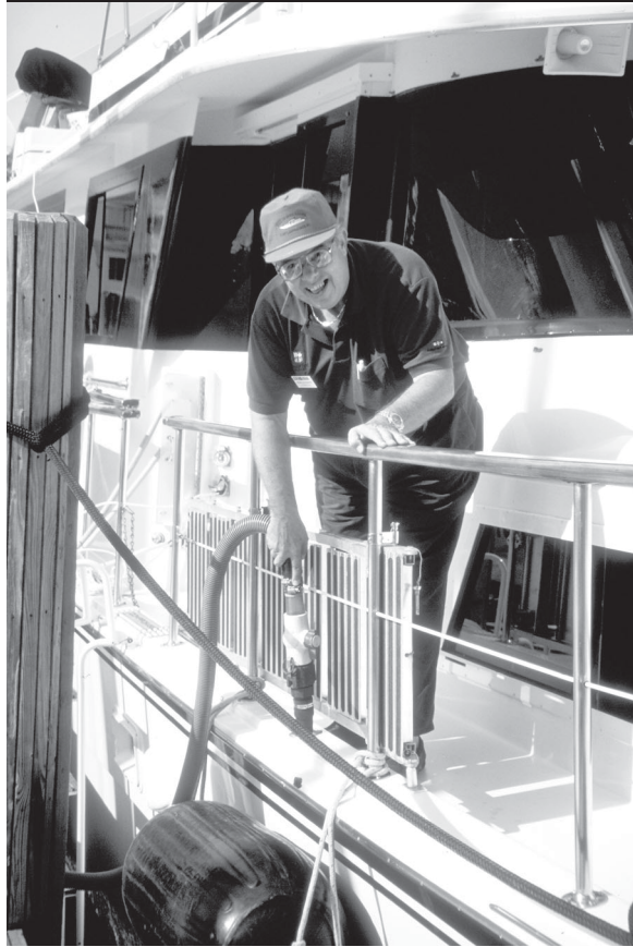
Figure 4-20. Pumpout system at Hall of Fame Marina (Florida). Accommodating dozens of yachts more than 100 feet LOA, the marina's pumpout system includes below-dock sewer pipes and connectors of each slip (USEPA, 1996: Clean Marinas—Clear Value ).
